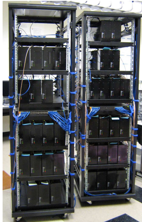
Figure 1: 39 of the testbed sites in two 42U racks
